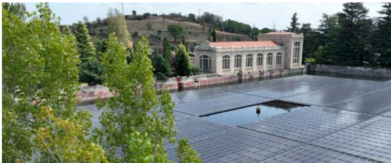
Picture 3. Floating photovoltaic solar plant in Torrelaguna (Madrid)
